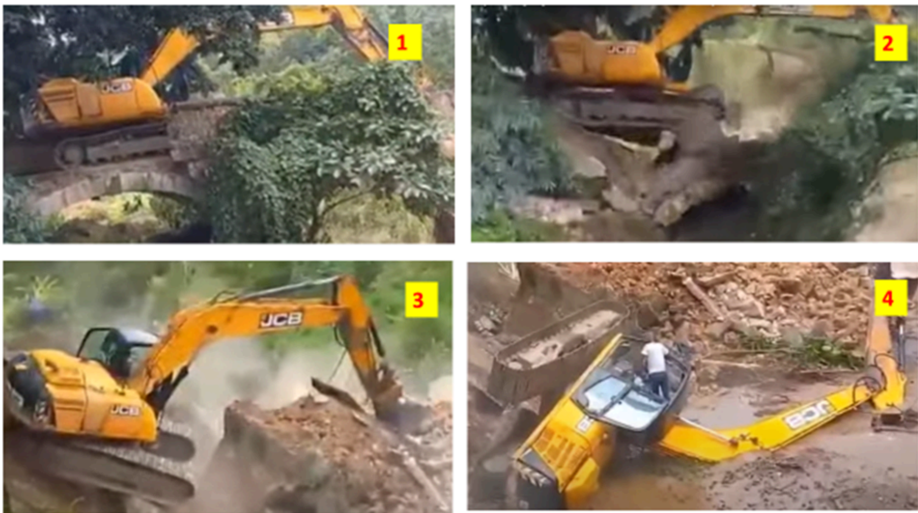
Figure 4. Sequence of the collapse of the arch and the excavator falling into the river. In image 3, the operator is trying to stabilize the unit using the bucket, however this is futile.
